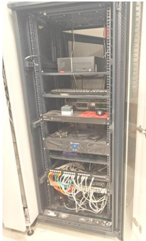
Armari rack elements centrals
